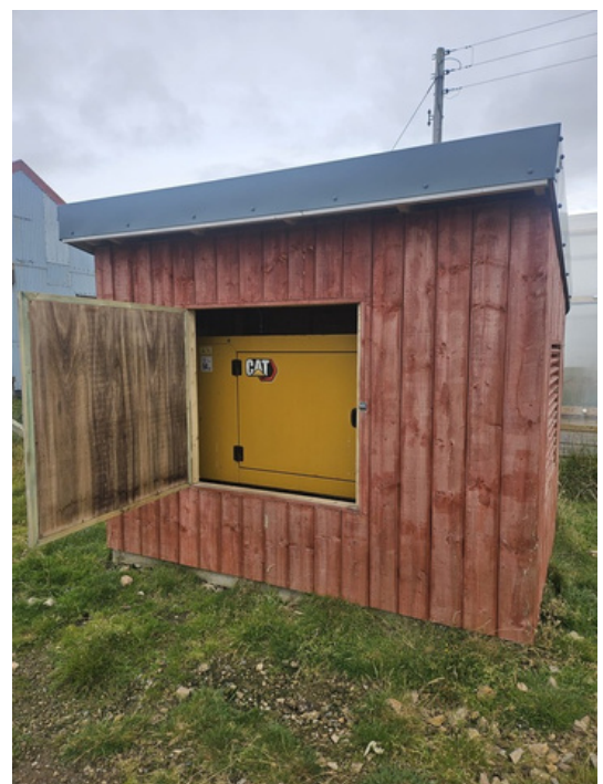
Sellafirth Hall generator
