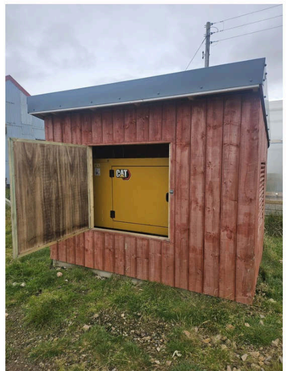
Sellafirth Hall generator
